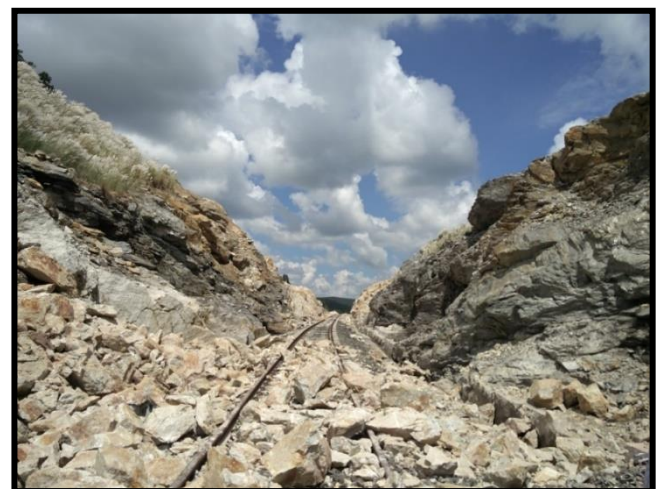
Figure 2 Initial condition of the slope
